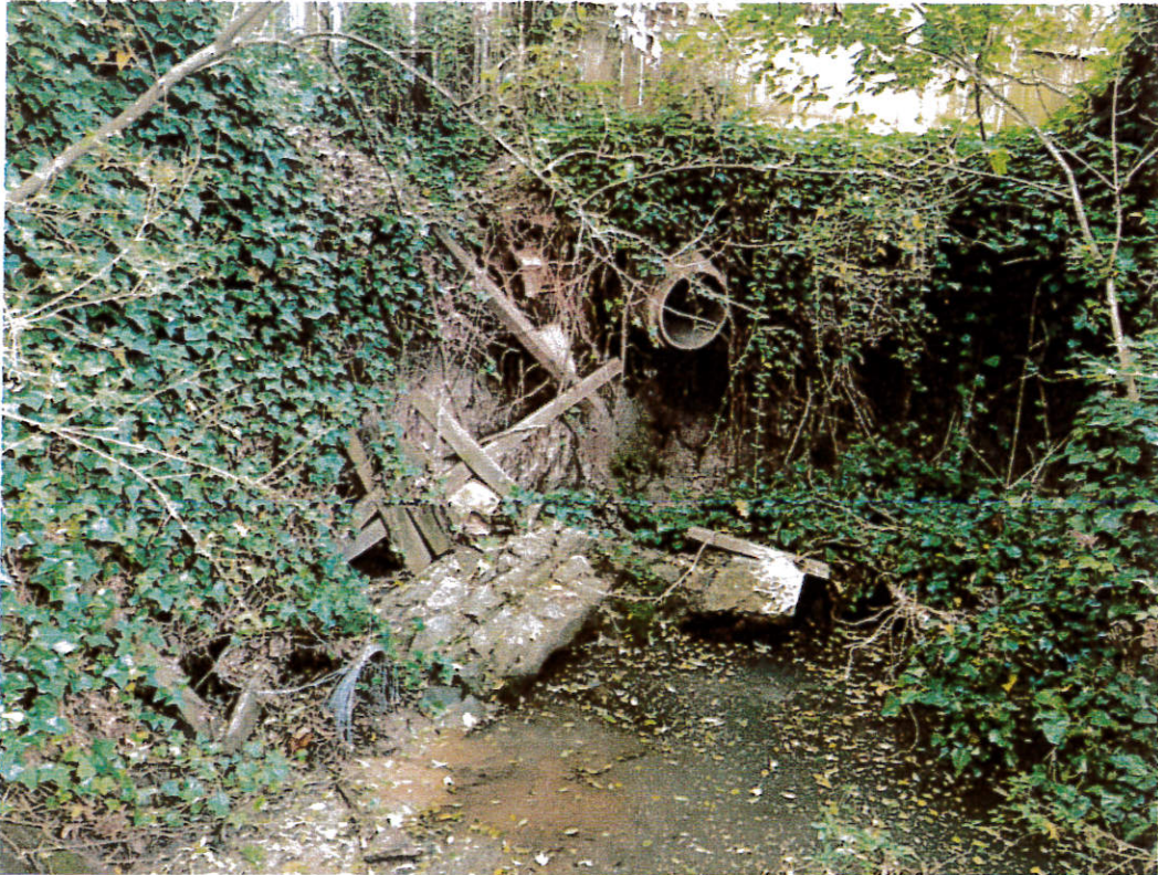
Beginning of stream – notice collapsed headwall and fence and eroded stream bank.
