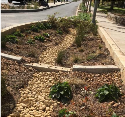
Green infrastructure – like this installation on McDonough Street – is an important part of Decatur's SWMP.
