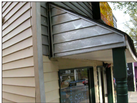
Vinyl siding is inappropriate on any commercial building in the City of Decatur.
