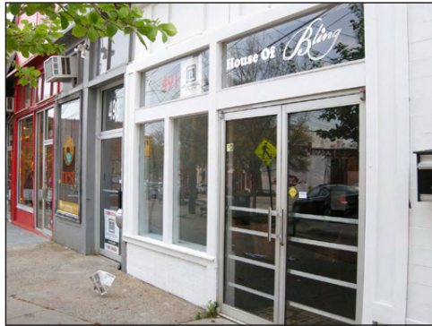
Commercial doors appropriate to the time period of the building should be retained.
