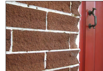
Sandblasting historic brick can destroy it as seen here.
