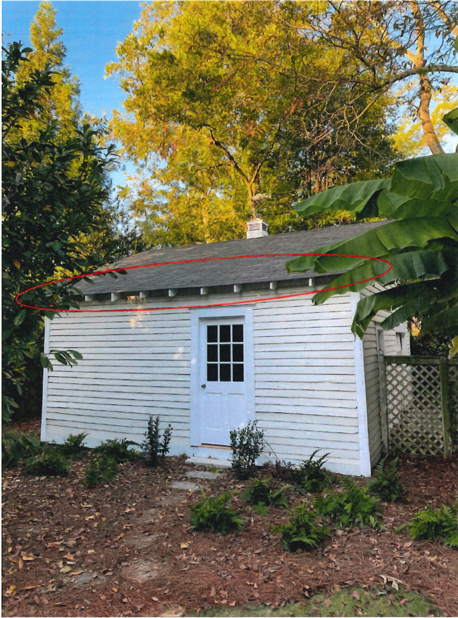
Detached garage roof line currently does not have any gutters (see areas circled in red).
